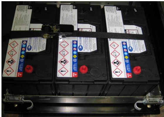
THREE GROUP 31 BATTERIES
