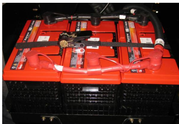
THREE ODYSSEY BATTERIES
