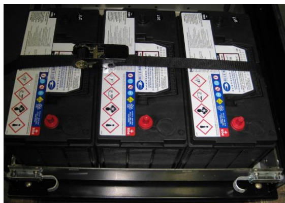
THREE GROUP 31 BATTERIES
