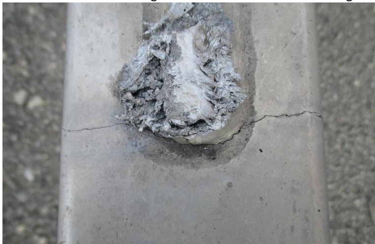
View of crack forming on underside of draft arm tubing
