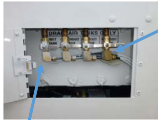
Wet Tank Drain Valve
