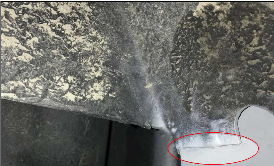
Figure 5. Reference photo of cut to air tank lower bracket.
