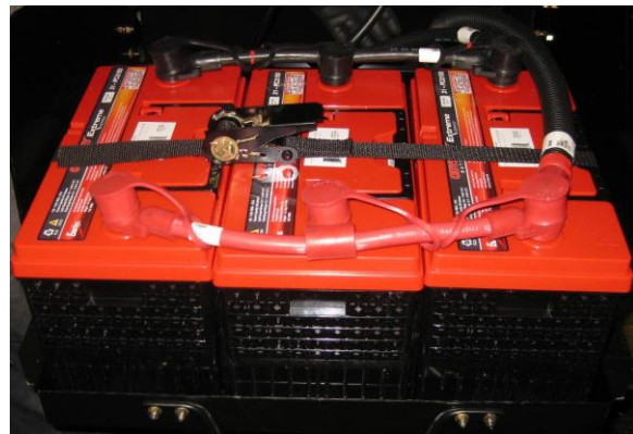
THREE ODYSSEY BATTERIES
