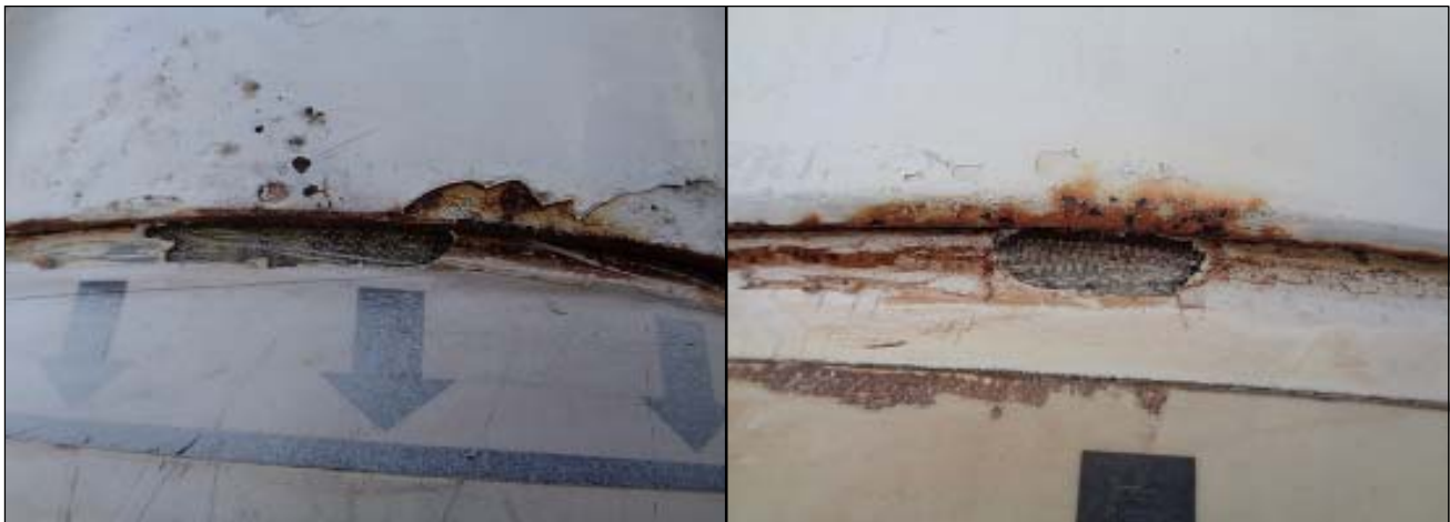
Figure 2 — Examples Of Gelcoat Damage
