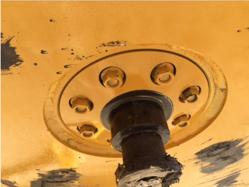
Improper Kingpin Installation
