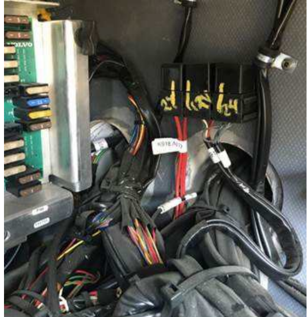
FIGURE 3: For vehicles not equipped with I-START dual battery system (until 3CET2V42XG5176275 ), find K918 at the right side of electrical distribution unit.
