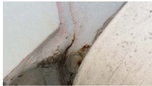
Paint crack that needs further examination
