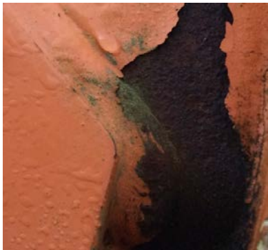
Rusty area needs cleaning to inspect
