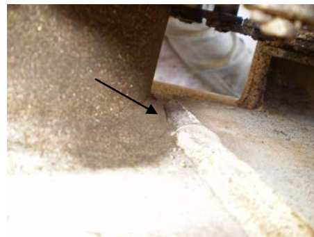
Crack at pivot inside boom
