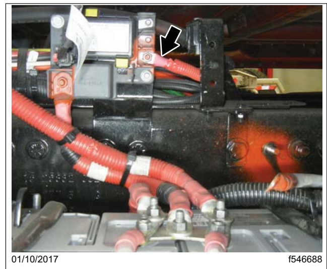
Fig. 28, CPDM Power Cable on the PNDB
