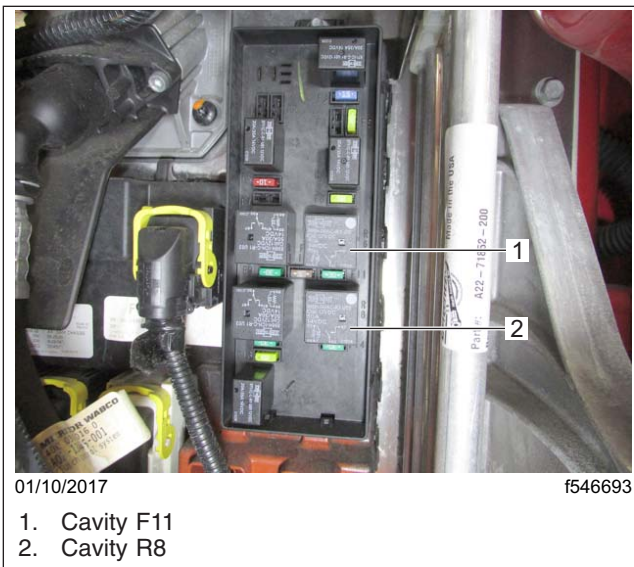
Fig. 34, Relays and Fuses on the SAM Chassis
