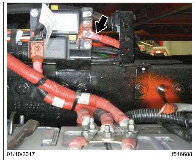
Fig. 28, CPDM Power Cable on the PNDB
