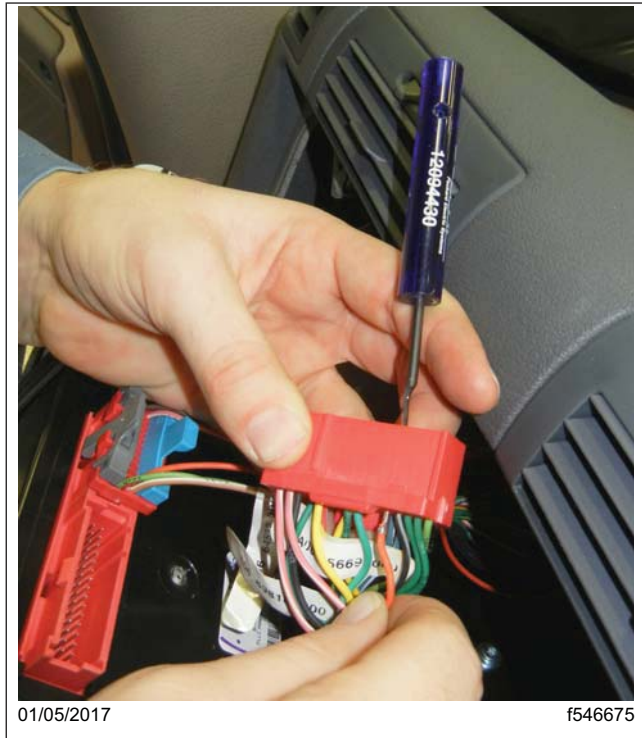
Fig. 15, Wire Removal from Cavity D12 of ICU Connector 2A
