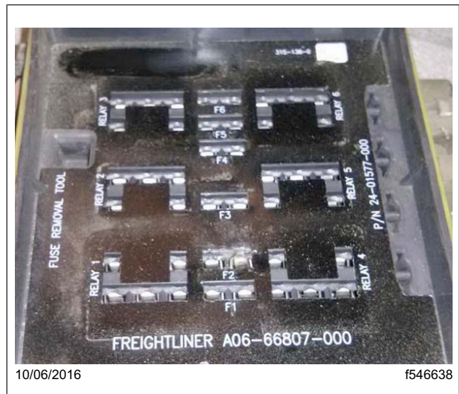
10/06/2016 f546638 Fig. 8, Incorrect: Heat damaged socket, debris accumulation
