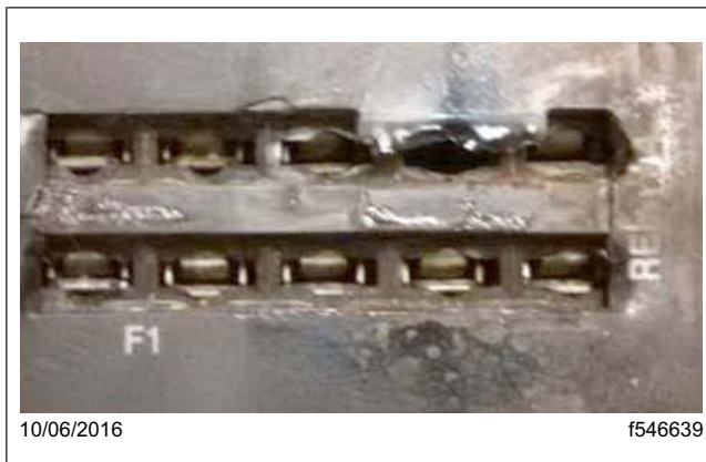
10/06/2016 f546639 Fig. 7, Incorrect: Heat damaged socket, debris accumulation
