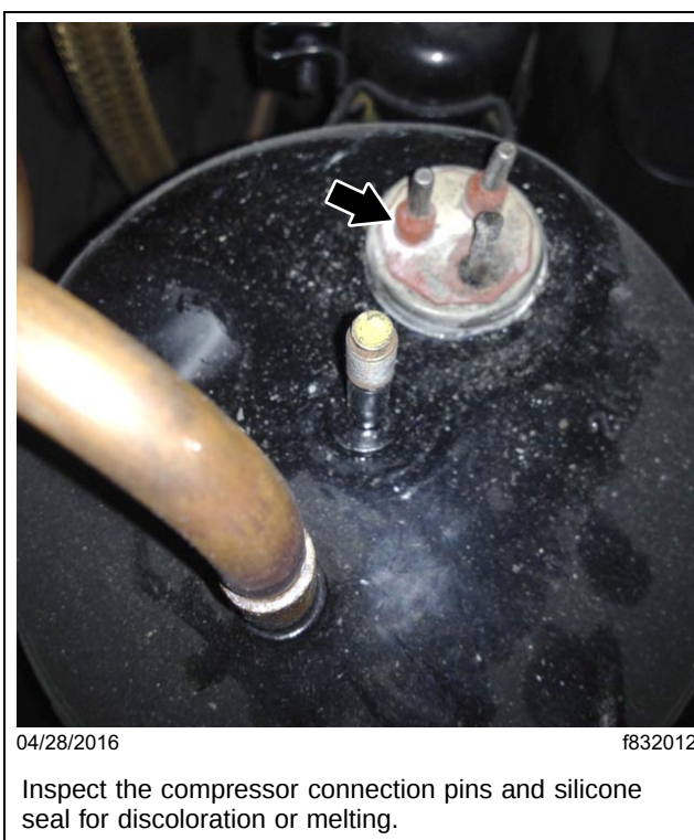
Fig. 11, Melted Silicone Insulator and Compressor Pin Damage
