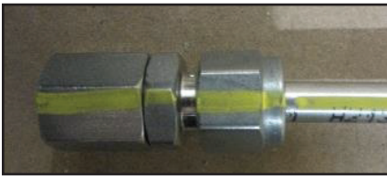
Figure 43: Yellow paint mark on the trigger line components.
