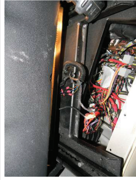
Wiring harness loose
