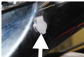
CHARGE AUX BATTERY (DIN)
