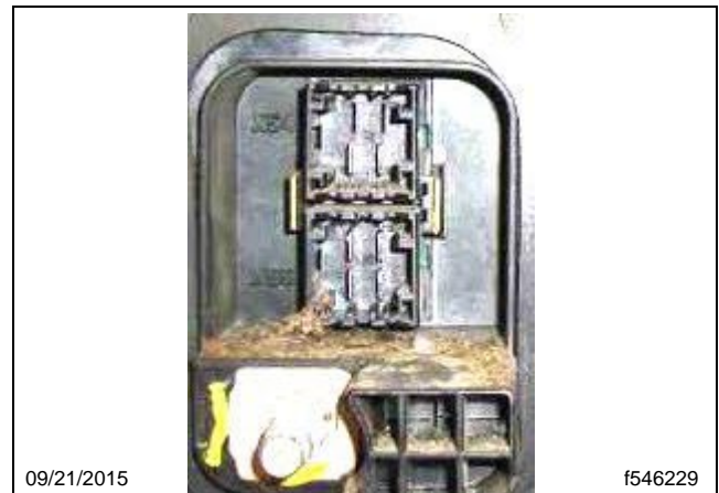
Fig. 6, Terminals with Dirt and Debris
