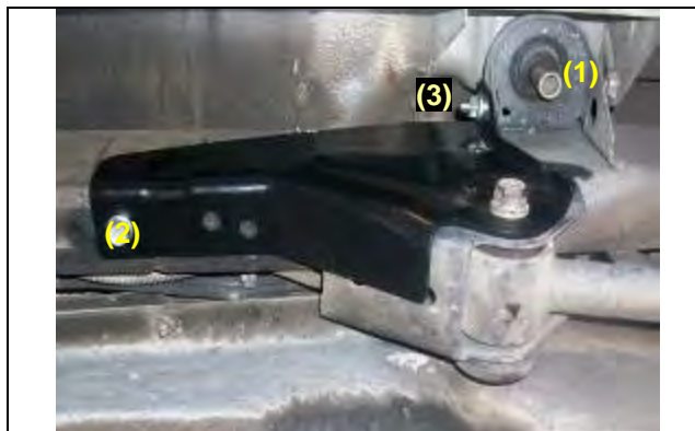
Figure 15 - Driver Side Temporary Installation 1. #4 Body Mount Lower Half Removed 2. Weld Nut Already in Frame 3. Stud and Nut
