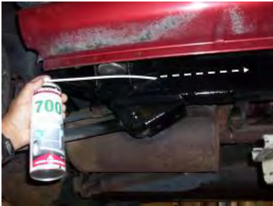
Figure 10 – Frame Hole Toward Front (300 mm)
