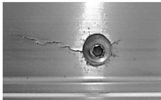
Figure 4: Spider crack on bottom rail
