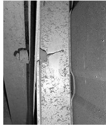
Figure 6: Crack on side post by front hopper slope.
