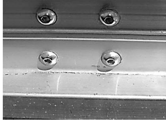
Figure 5: Crack on the top inside corner of bottom bulb.
