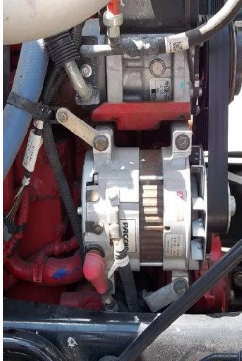
Figure 1 – Positive cable goes DOWNWARD, OK , no further action required
