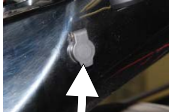
CHARGE AUX BATTERY (DIN)
