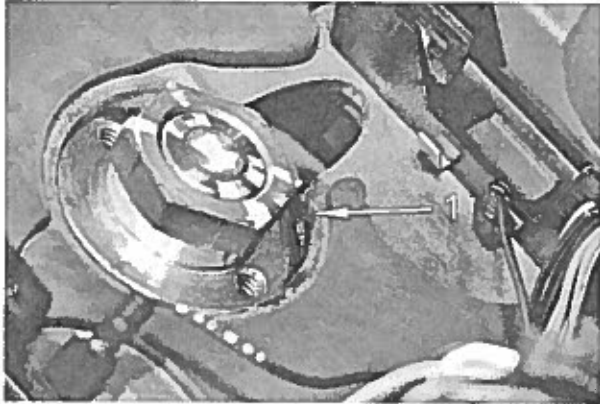
Figure 3 1 Gap between center hub and outer ring.
