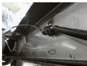
Wiring properly placed in P-clamp.
