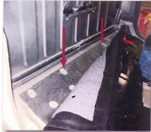
View of suspect inboard seat belt anchor locations with floor covering pulled back
