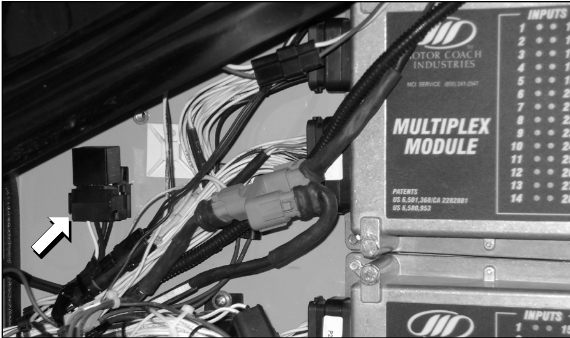
Figure 14. Front junction box compartment.
