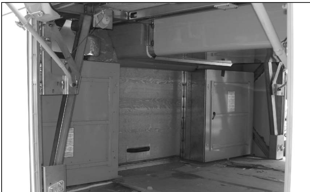
Figure 31. #3 baggage bay compartment.
