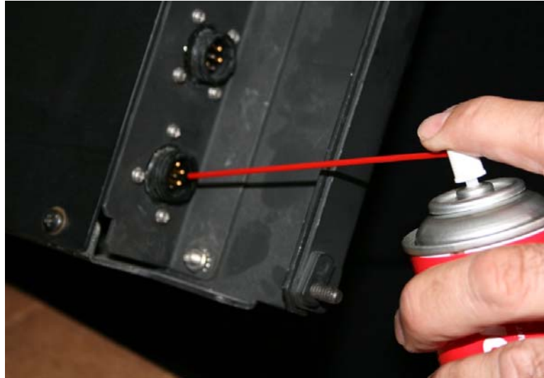
Fig. 2 Spray Corrosion X in unused connector
