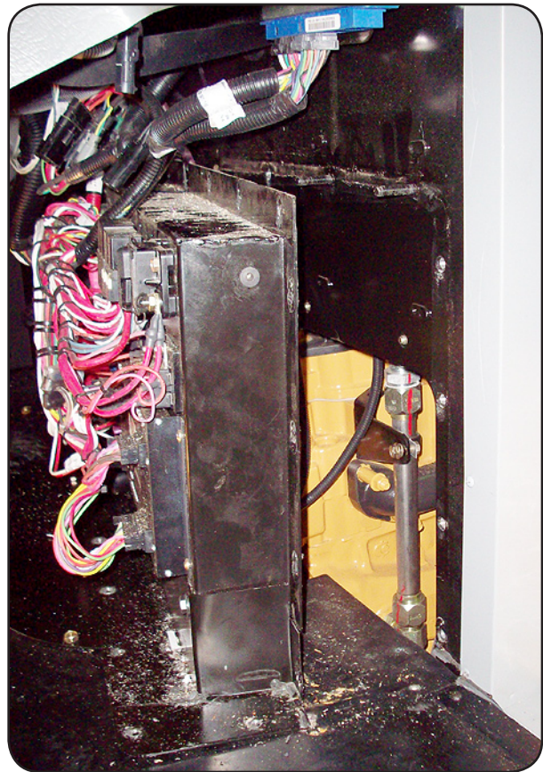
PDU pulled outward at right side to gain access to cables at rear of engine
