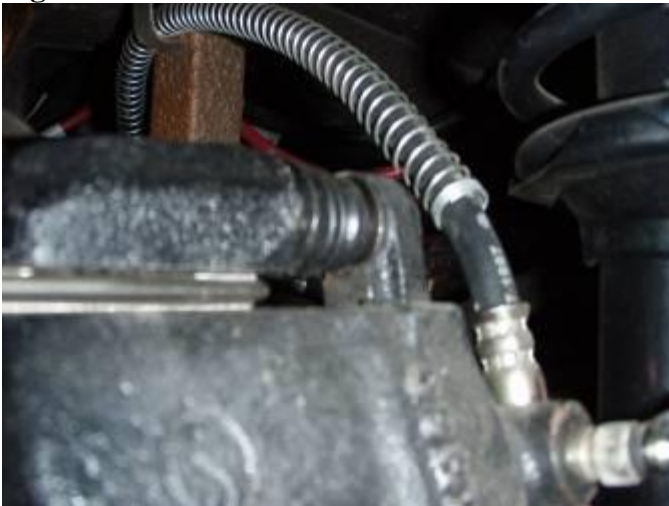
Figure 18. Brake Slide Bolts
