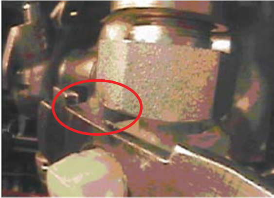
A gap exists between the pipe flare nut and the stay with no interference.
