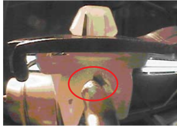
A gap exists between the pipe and the clip.
