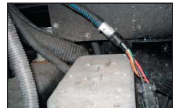
Figure 1B Wiring harness shown has adequate clearance.
