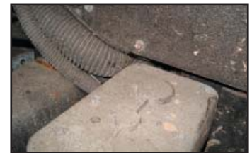
Figure 1A Wiring harness shown requires repairs identified in this bulletin to allow adequate clearance.
