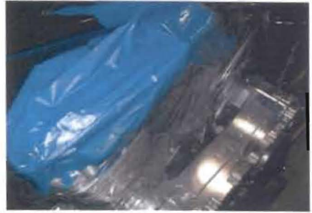
Photograph showing protective covering on the motor and primary
