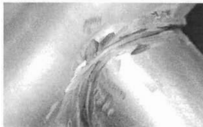
Carefully remove the original weld. And prepare the joint per the illustration to the right
