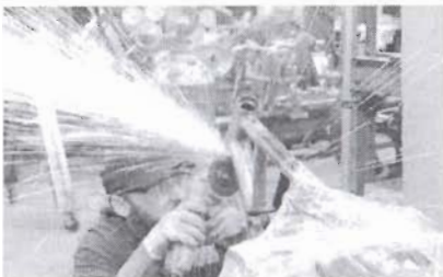
Using a thin grinding wheel remove the existing weld around the joint
