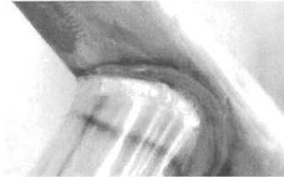
Photo of a concave/undercut 2 nd pass, requiring third weld pass
