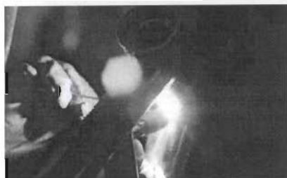
Using TIG process and a .062" ER70 rod to complete the third pass
