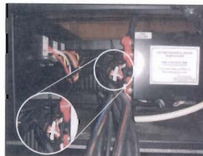
Figure 4 In-line fuses secured off compartment floor with wire ties
