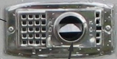
Typical furnace exhaust vent.
