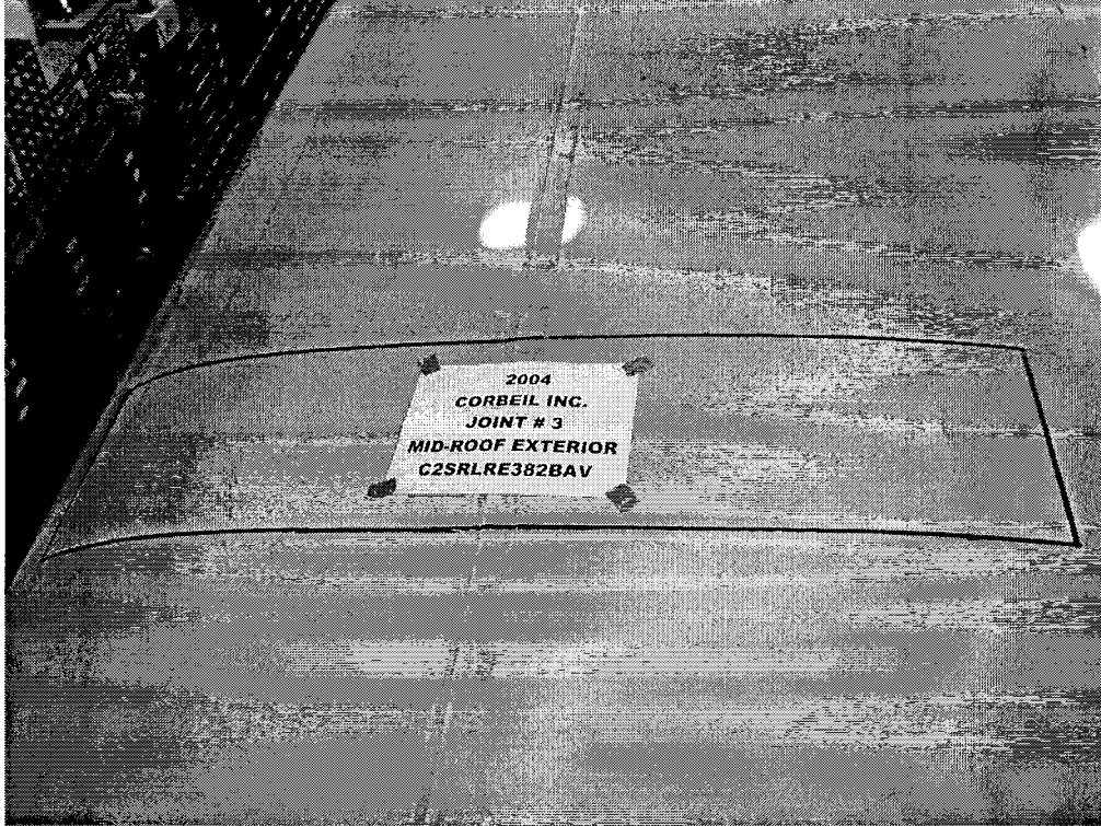
Joint #3 Corbeil longitudinal roof joint
