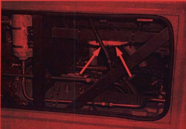
Figure 7: T2145 - Behind the RH engine compartment side door - engine compartment to central tunnel line connection. Check two crimp fittings.
