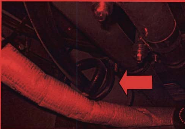
Figure 11: Spare line duct at the front of the coach with new central tunnel line installed
