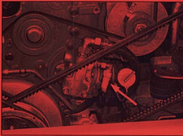
Figure 5: Behind rear engine compartment door - C2045 and T2145 w/ Detroit Diesel engine - pressure feed line at hydraulic pump. Check one crimp fitting.
