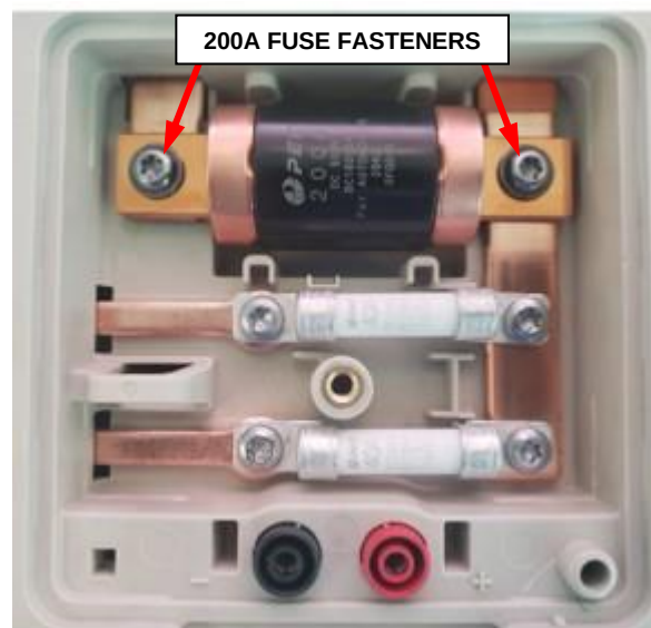
Figure 8 – 200A Fuse Fasteners
