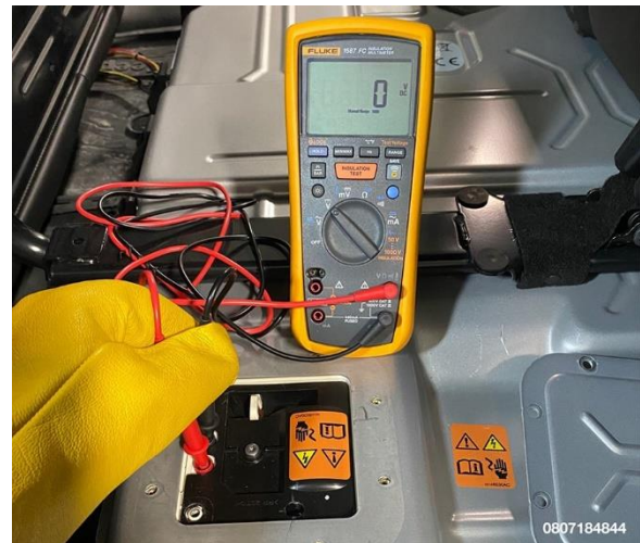
Figure 6 – Measuring at High Voltage Test Points
