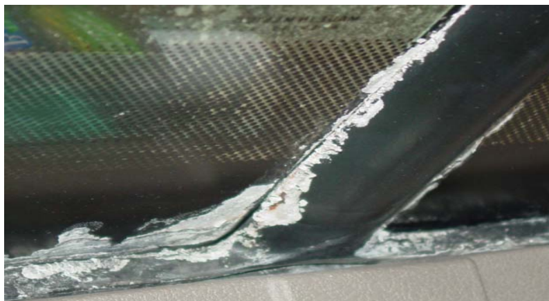
White residue (road salts) indicating leak between windshield seal and glass.
