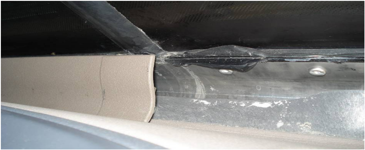
Residue trail indicating leak between windshield seal and glass and/or leak in windshield seal adhesive.
