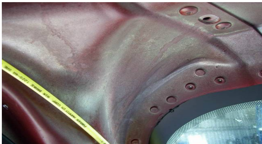
Signs of water coming in through leak in roof-cap joint and dripping down A-pillar.
