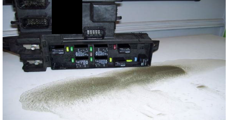
Water inside module
