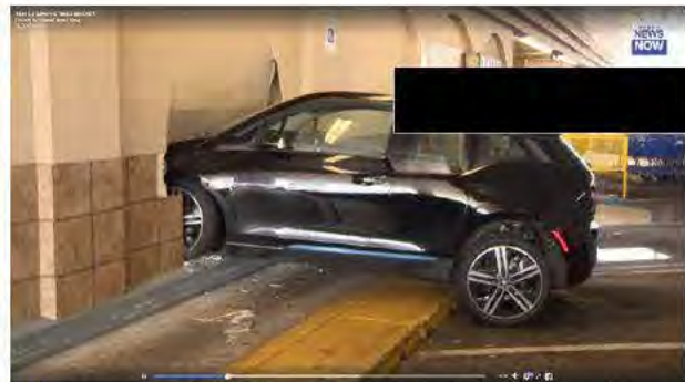
Figure 32. Side view showing damage to the wall behind the parking space. Store entrance is in the background. 47
