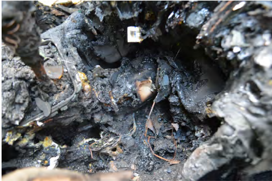
Figure 3: The Area of Fire Origin
