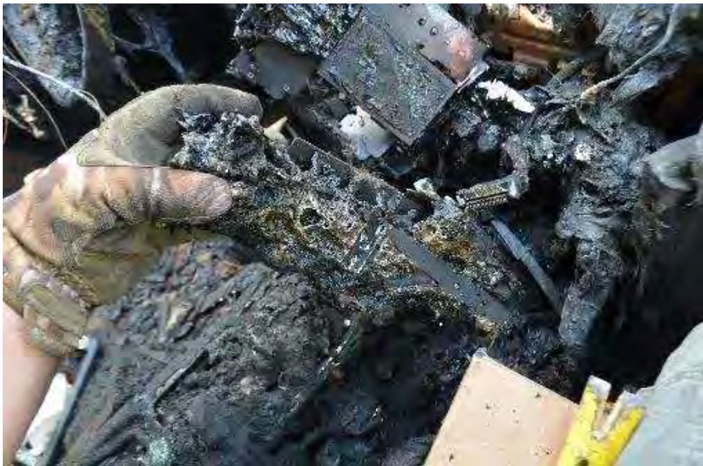
Photograph 8: The severely fire-damaged air conditioner controls.
