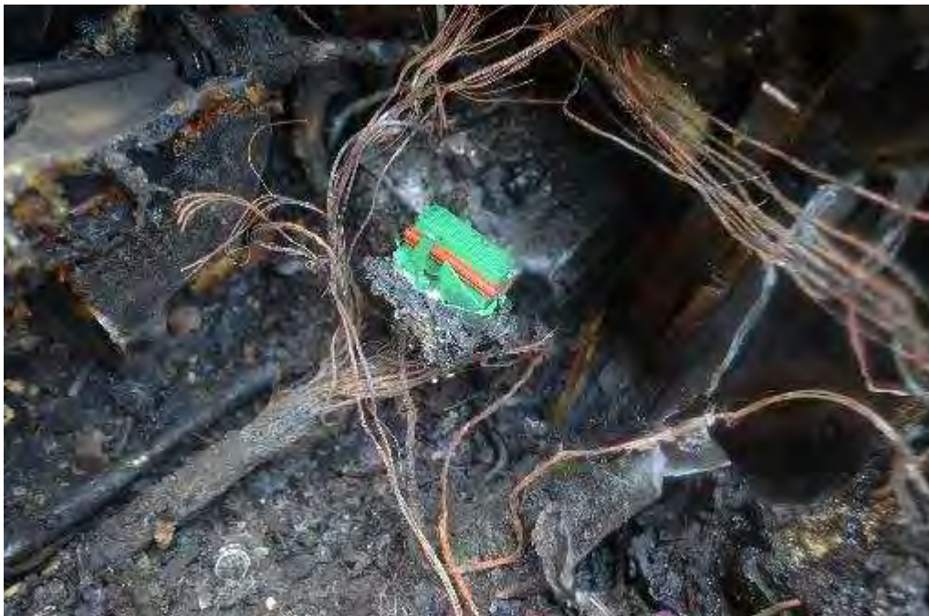
Photograph 10: Electrical conductors in the area of fire origin, with no sign of fire-initiating failure.
