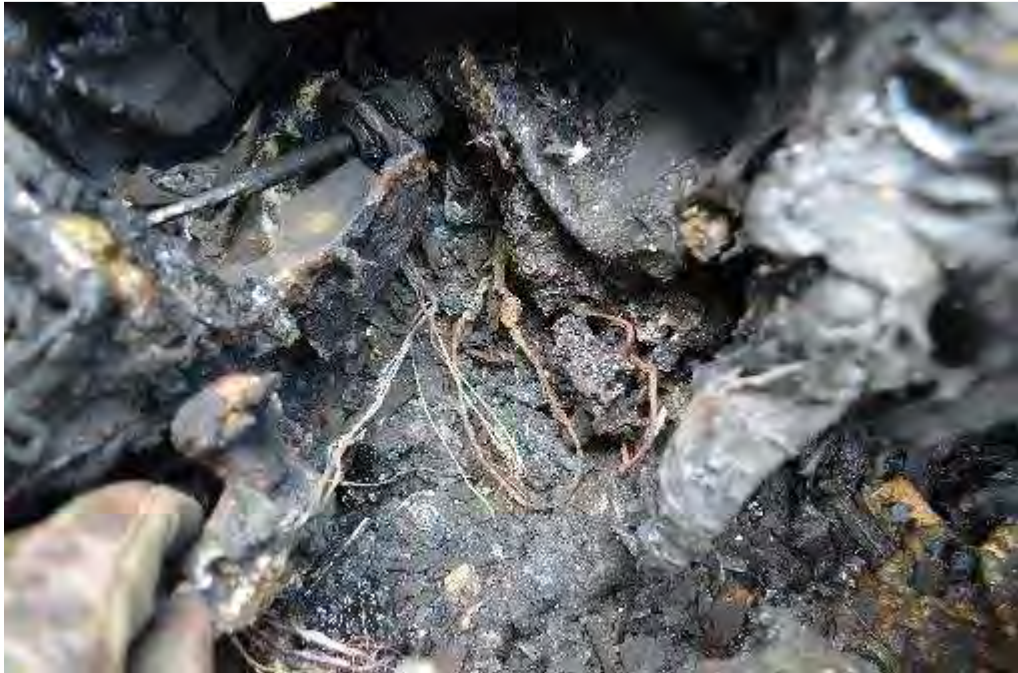
Photograph 9: Electrical conductors in the area of fire origin.
