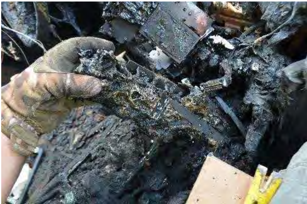
Photograph 8: The severely fire-damaged air conditioner controls.
