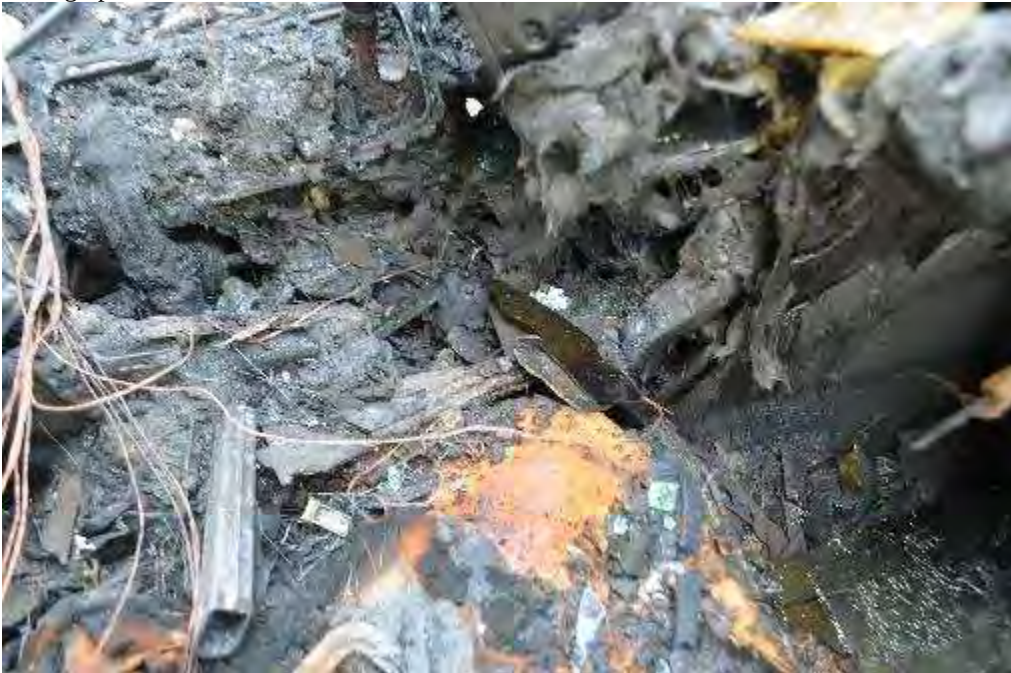
Photograph 6: The base of the dashboard and console. The area of fire origin.
