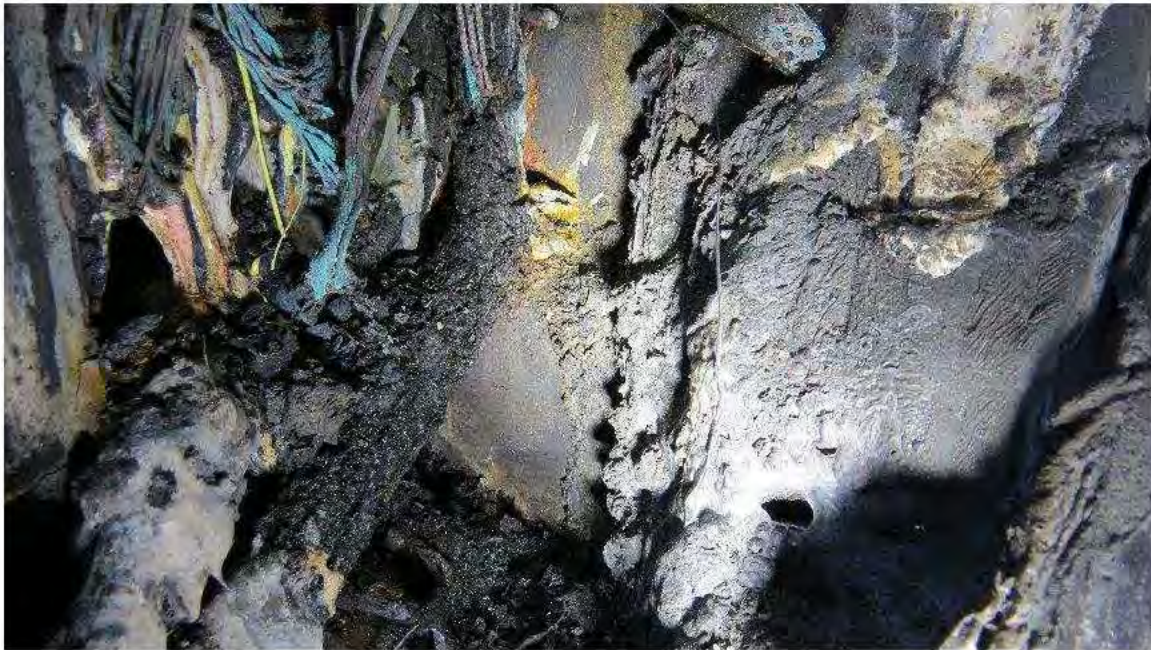
Photograph 10: Fire-damaged OEM cables in the bottom of the driver's side kick-panel.
