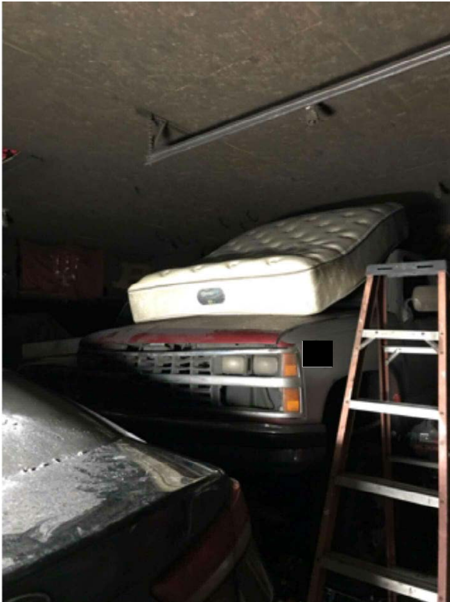
Damage to the osb
