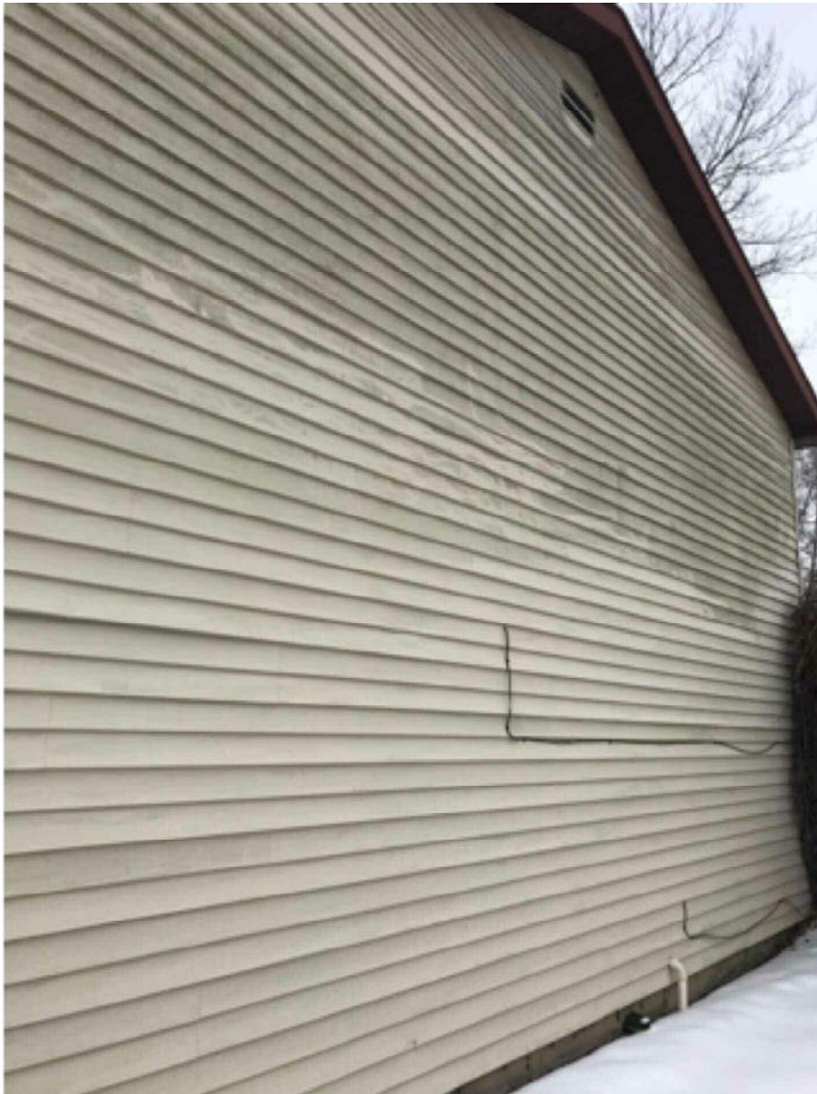
Soot in siding
