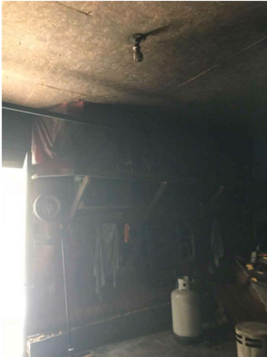
Garage. Electrical affected
