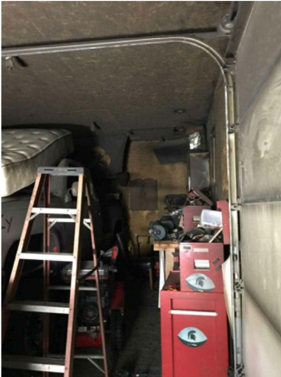
Damage to the osb
