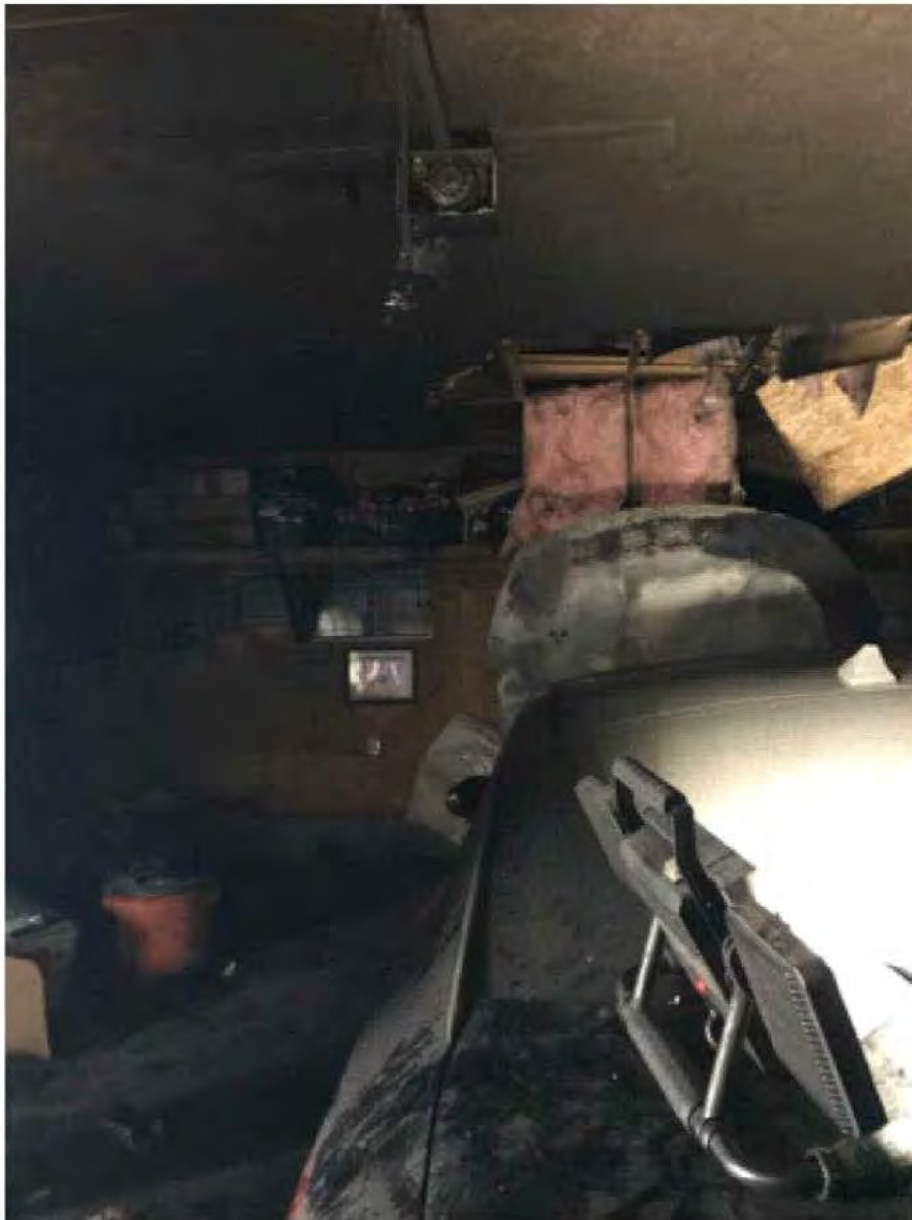
Melted garage door opener
