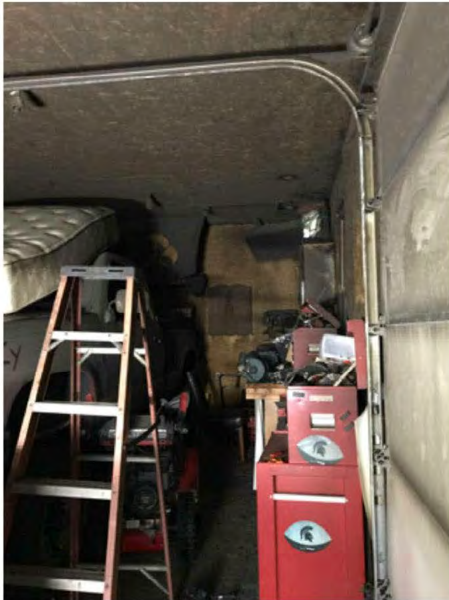
Damage to the osb
