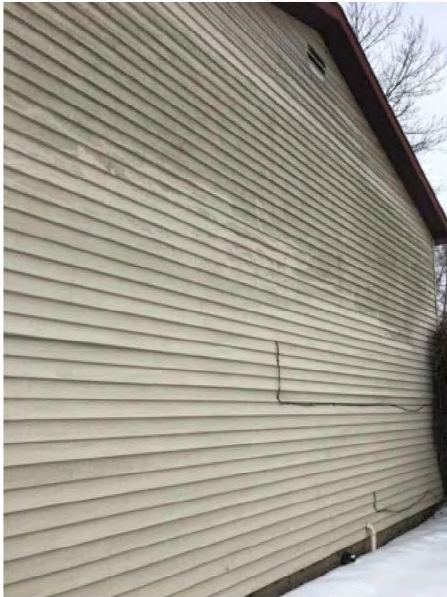
Soot in siding
