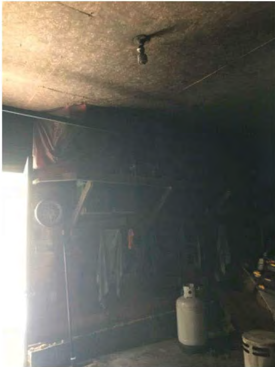
Garage. Electrical affected
