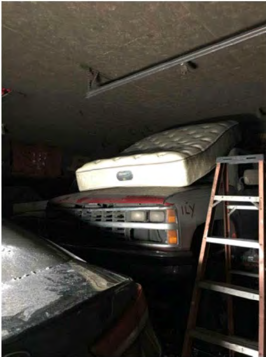
Damage to the osb
