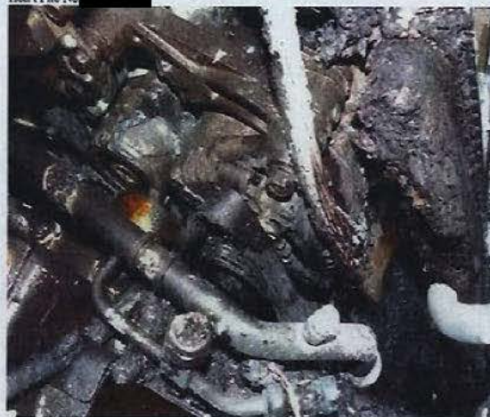
41. View of the alternator, right front.
