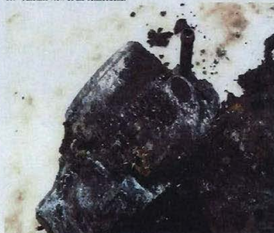
10. Another view of the connections.
