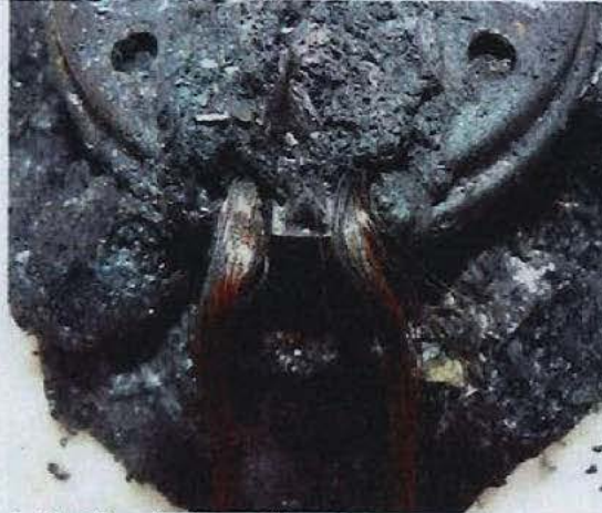
7. View of the cooling fan motor wiring connector.
