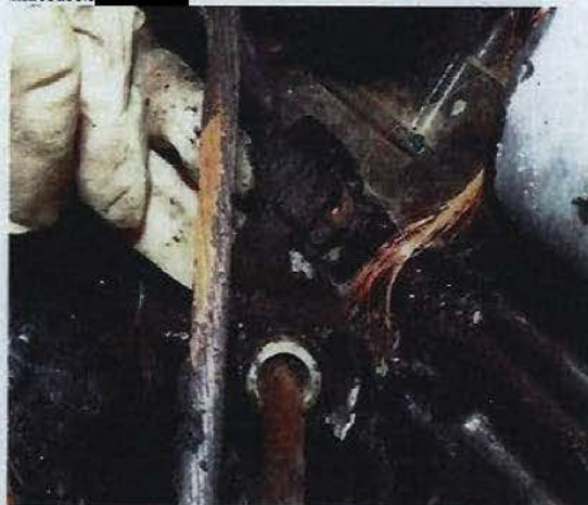
35. View of the starter cable connection.
